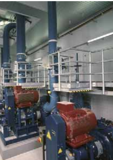
Maschinensatz Abwasserpumpwerk Machine unit of sewage pump station
