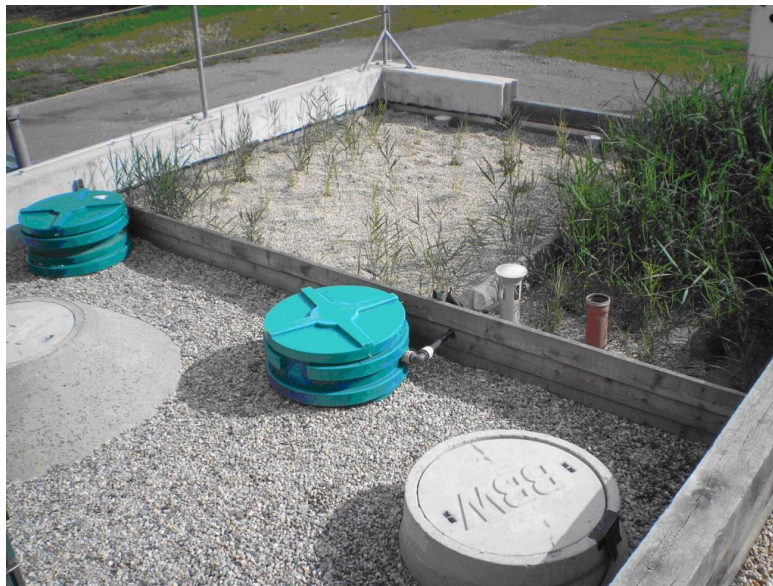
Figure 23: Constructed wetland Type UFZ C+H 4 E: photo of the Demobox BDZ in Leutzsch
