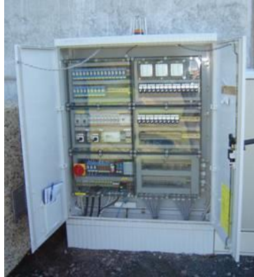
Figure 7: Siemens S7-200 PLC outside the Demo Box building
