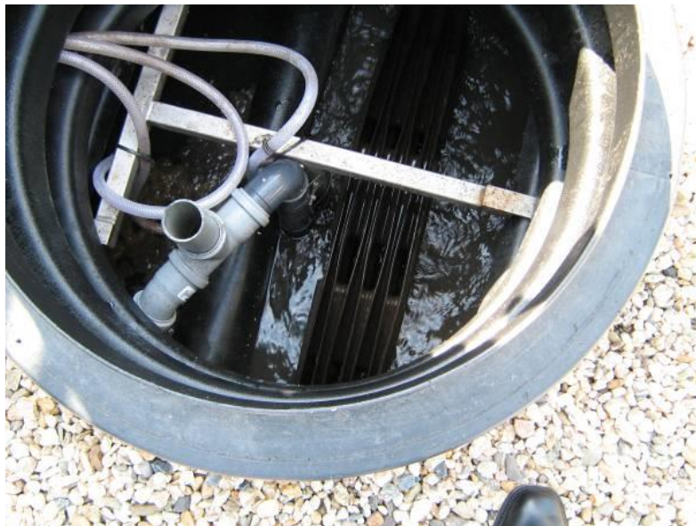
Figure 10: Photograph of the system in operation (BDZ Leipzig)
