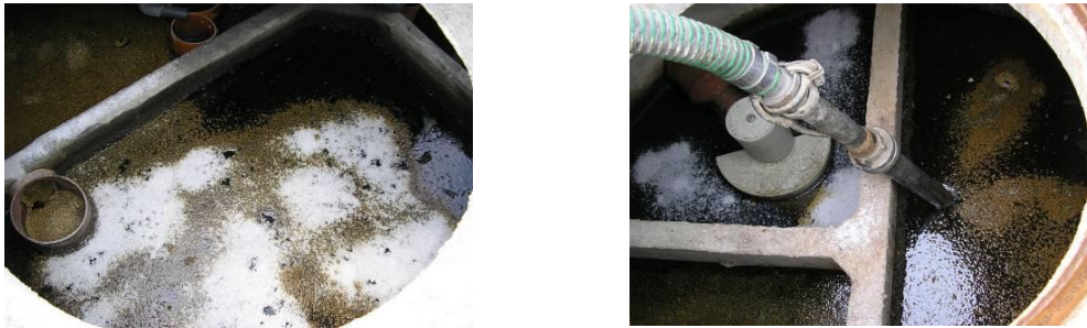
Figure 43: Oil accident: An oil-binding agent was applied and suctioned out of the primary clarifier.
