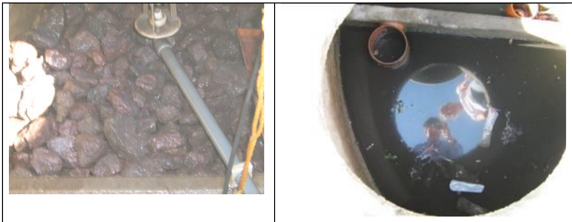
Figure 17: Trickling filter KP253 PAL and primary treatment (BDZ Leipzig)
