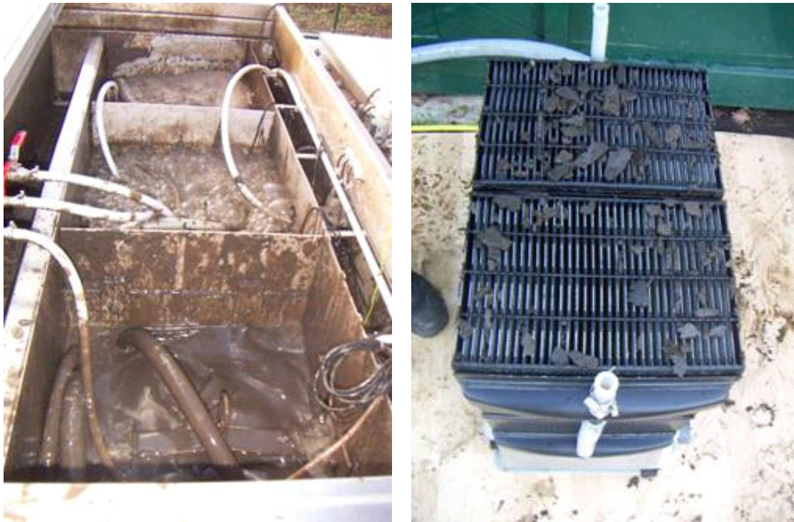
Picture 6 Reactor thickening and module clogging
