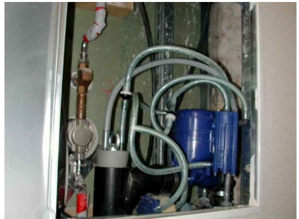
Vacuum control valves
