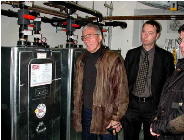
Urine tank facility (picture made during press presentation)
