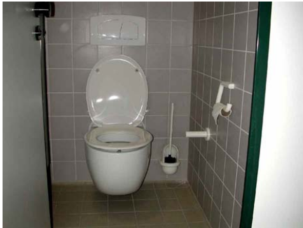
Gravity separation toilet
