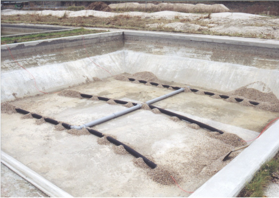
Figure 36: Drainage pipes on the basis of the slow sand filter during sand exchange.
