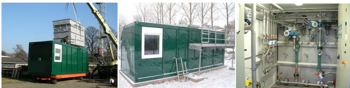
Figure 11. Container plant (incorporation of biological reactor, after construction on site and machine room)
