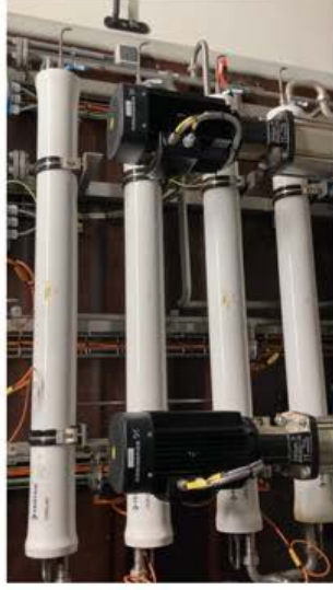
Reverse osmosis membranes
