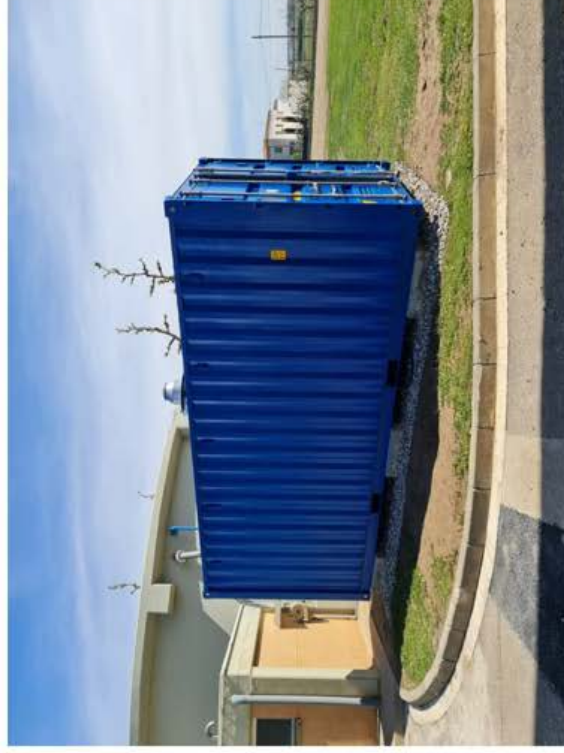
SOFC pilot plant installed in WWTP Lleida
