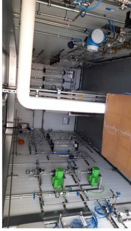
What has been done: real picture of the SOFC pilot plant (taken April 2022)
