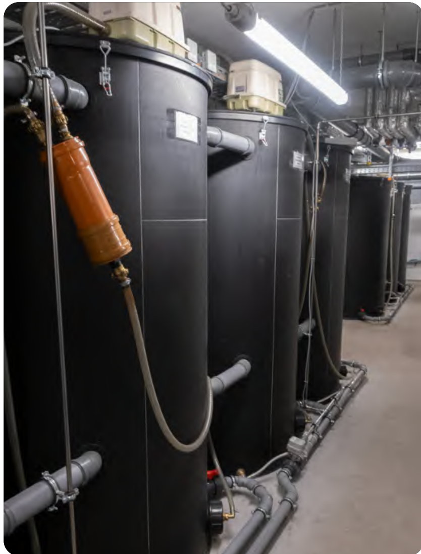
Greywater recycling system in a Berlinovo student apartment complex
